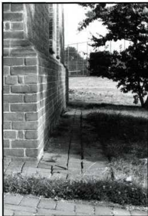
A foot-wide extension of bricks catches runoff from the roof of the science building, reducing erosion around the base.
