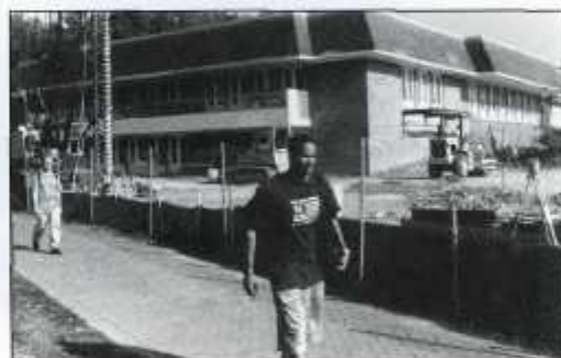
Charles Hall begins its growing pains. Construction will double its size and greatly enhance its facilities.
