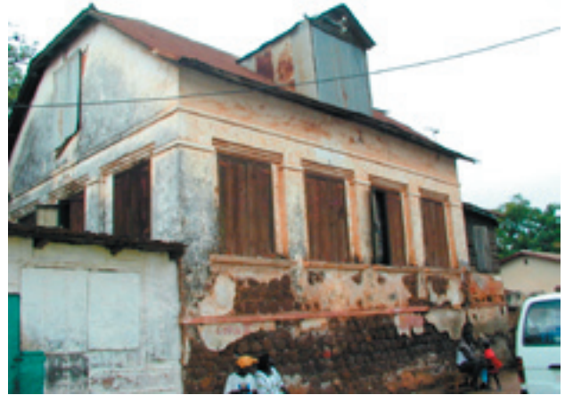
An example of a block house that currently is in a poor state of repair. Many of these older houses are likely to disappear in the future because the cost for renovation is so expensive.
